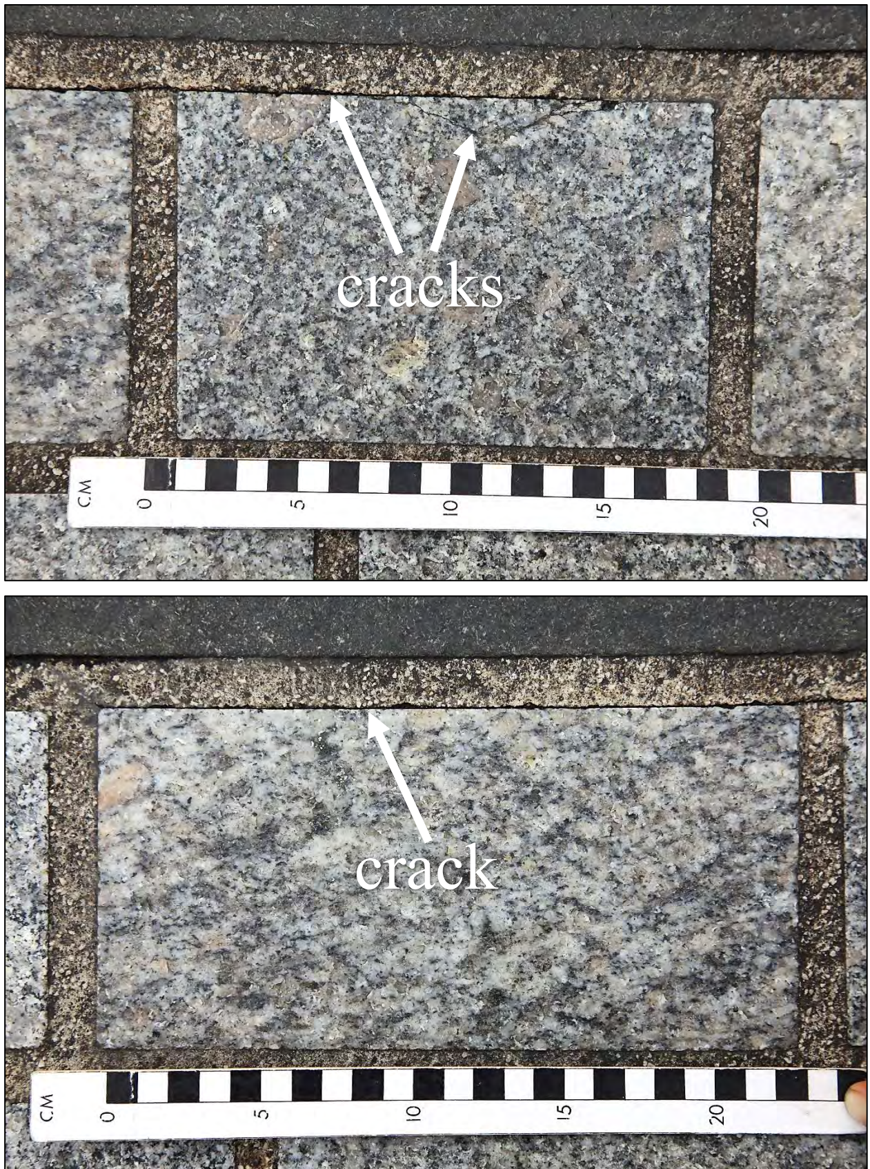
Figure 10 Performance issues in a recently setted area at Waverley Bridge
