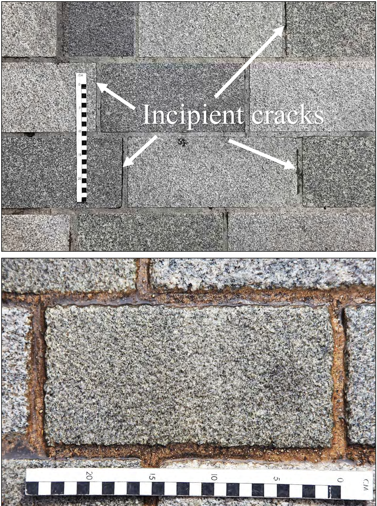
Figure 9 Performance issues in recently setted areas at St John Street and New Street
