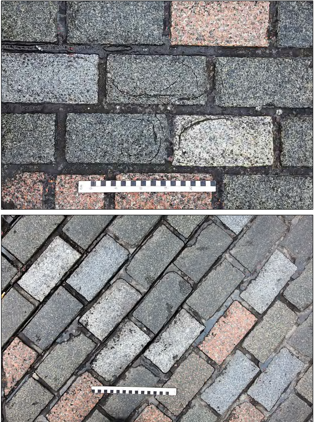
Figure 8 Performance issues in a recently setted area at the junction of South Bridge / North Bridge and Royal Mile
